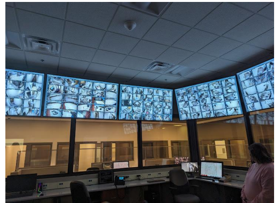
Main Control Room, partial
