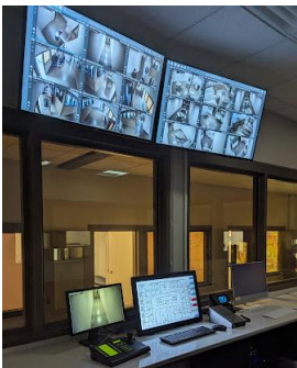
Individual hall monitoring
